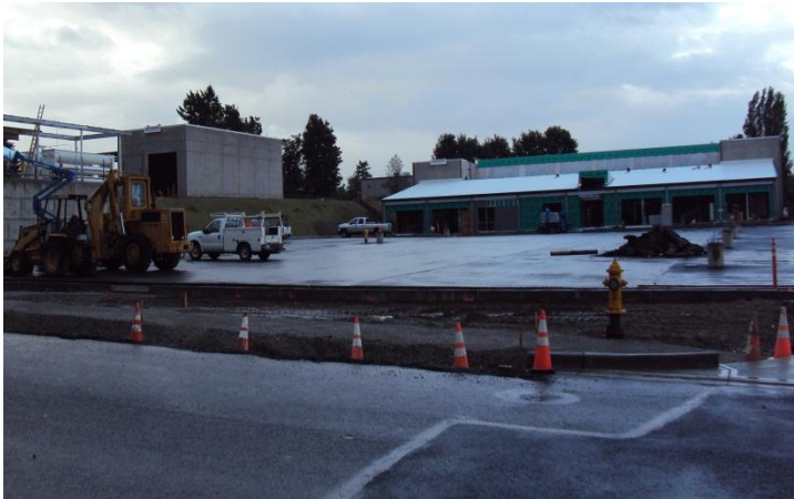
L to R: CNG Storage Tanks, Bus Wash, Bus Maintenance Building
